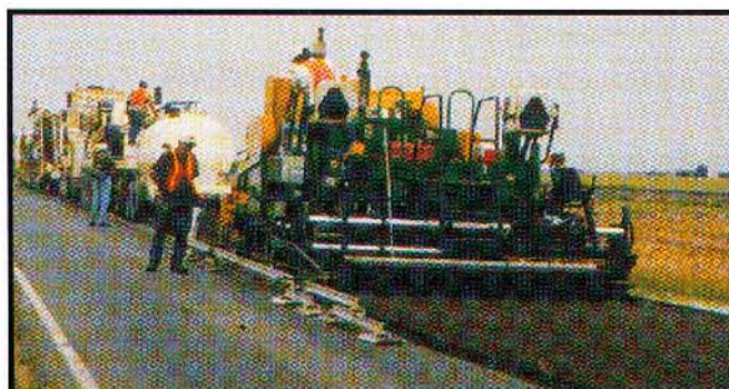
The new surface is laid and compacted; a fog seal may be applied following final compaction.
