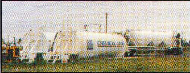
Lime slurry is manufactured on the job site with PORTA BATCH® mobile lime slurry production units provided by CLC.
