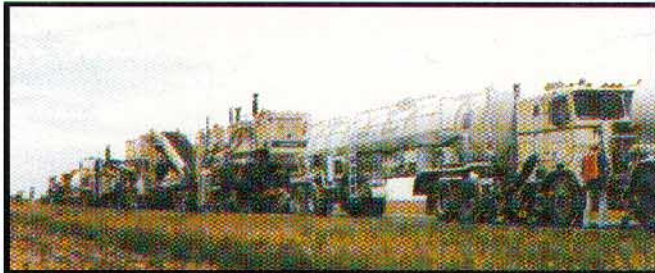
Old asphalt pavement is removed and processed with lime slurry and asphalt emulsion in the recycling "train."
